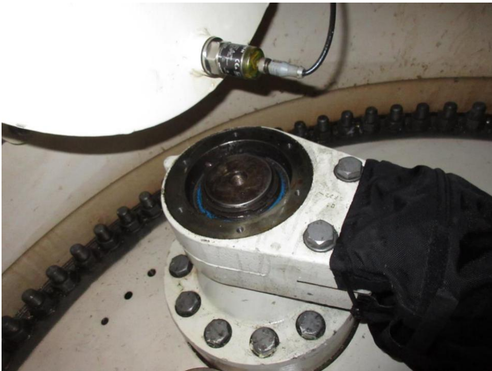
Overview link bearing of the pitch systems
